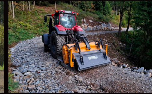
RC90 Stone crushing
